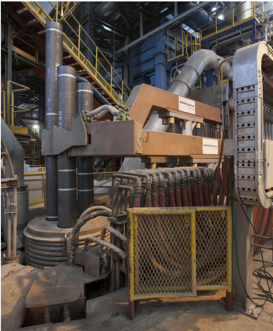
Twin-ladle furnace built by SMS group.
