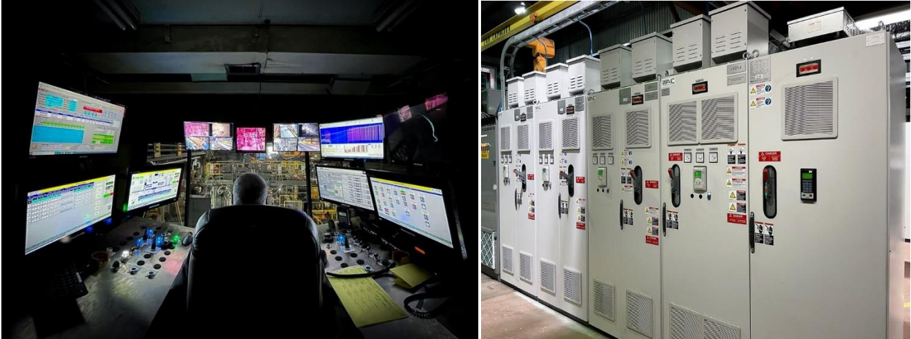
Figure 1,2 – Main pulpit and new electrical panels.
